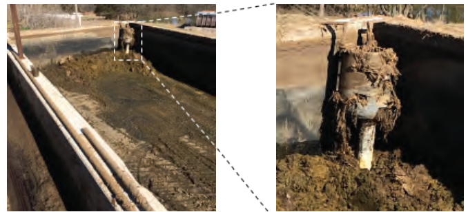
Figure 8a and 8b. PPSB with liquid discharge pipe (left) and discharge pipe (right).
