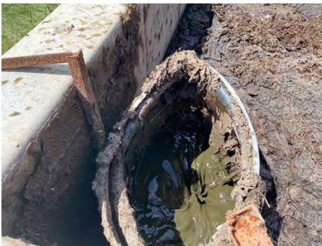
Figure 8d. Water discharging from the PPSB.
