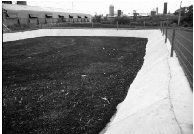
Figure 1. A concrete-lined earthen pit may allow the use of steeper side slopes, which decreases the area required per unit of storage volume. It also provides a more pleasing appearance.
