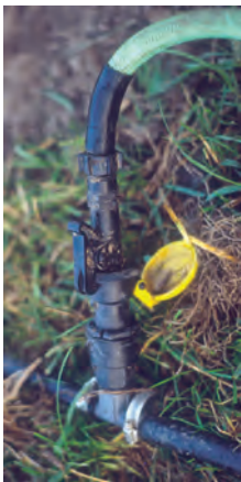
Figure 13. Quick-attach valve for a portable water system.
